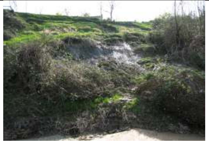
Sloughing of the slope near the North delta ravines.
